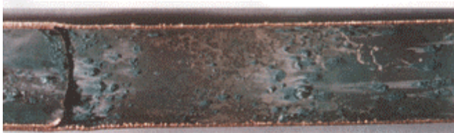
Internal corrosion (Photo: CEBTP)
